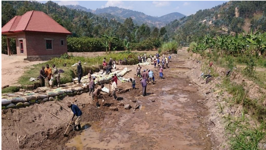
Figure 64: Diversion channel under construction (for excess flow from Karimo and Gisunyu rivers)
