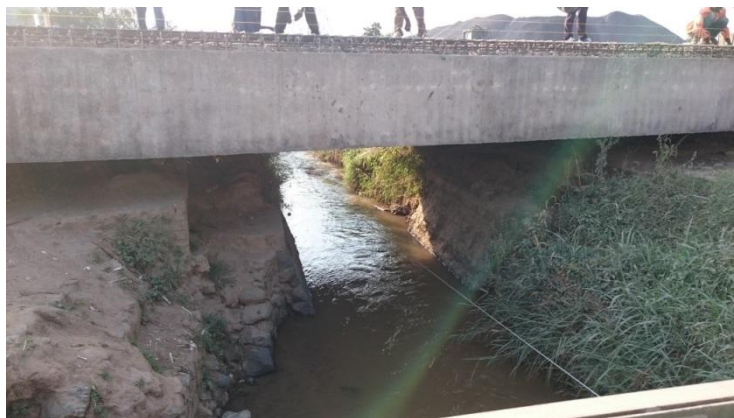
Figure 3 New bridge on river Pfunda: former bridge has not been destroyed, potentially hampering peak flows
