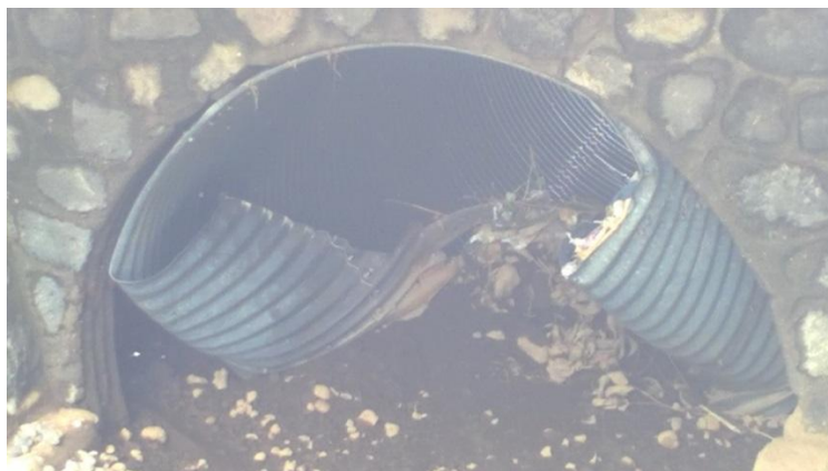
Figure 4 Muhe river bridge (view from upstream): corrugated metal pipe severely damaged (repaired in meantime)
