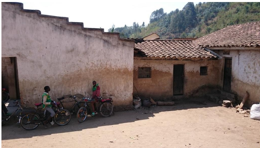
Figure 63: Confluence of Karambo and Gisunyu (right bank): high water mark on 3 rd generation houses
