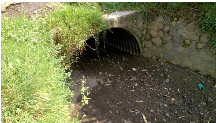
Figure 39: Partially blocked culvert on river Susa (main road to military academy)
