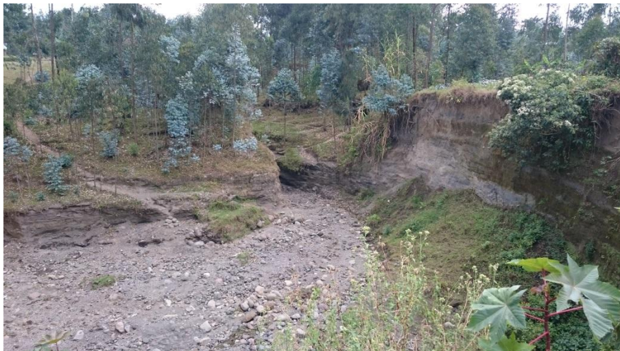
Figure 115 Threatened embankments requiring lateral protections
