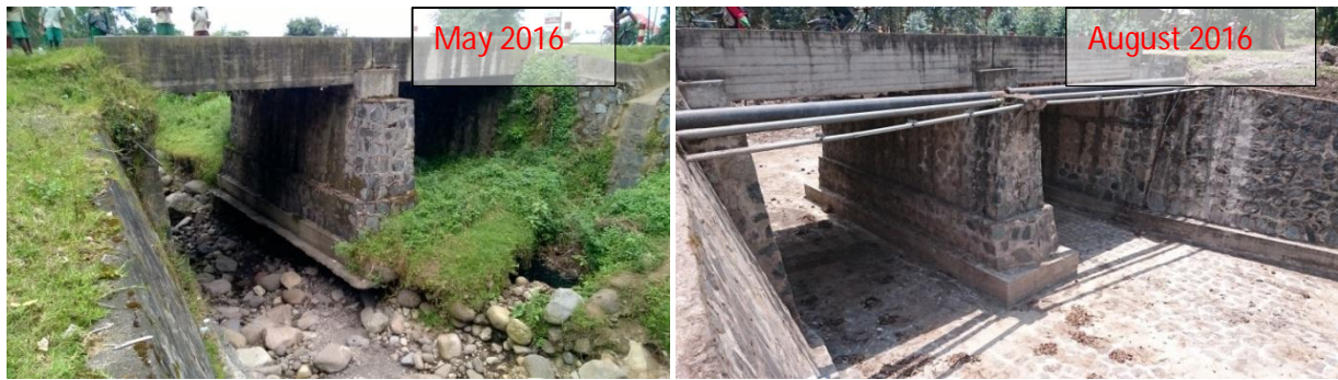
Figure 2 Example of efficient maintenance works on river Rwebeya (Bridge on RN2 road from Musanze to Kinigi)
