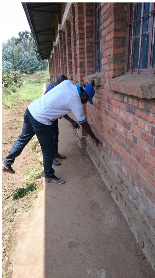
Figure 75: School Saint Matthieu: school's warden indicates high water mark
